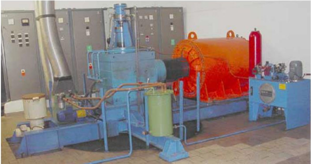
Fig. 1. Hydrogenerator of small hydropower.
