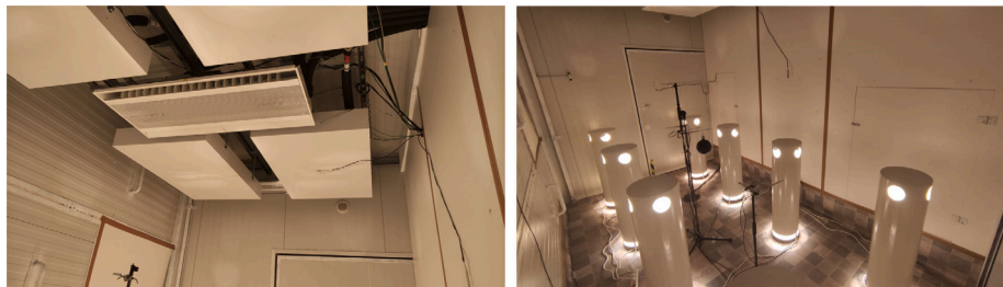
Fig. 11. Measurement of ceiling cooling system in IDO part of CC.
