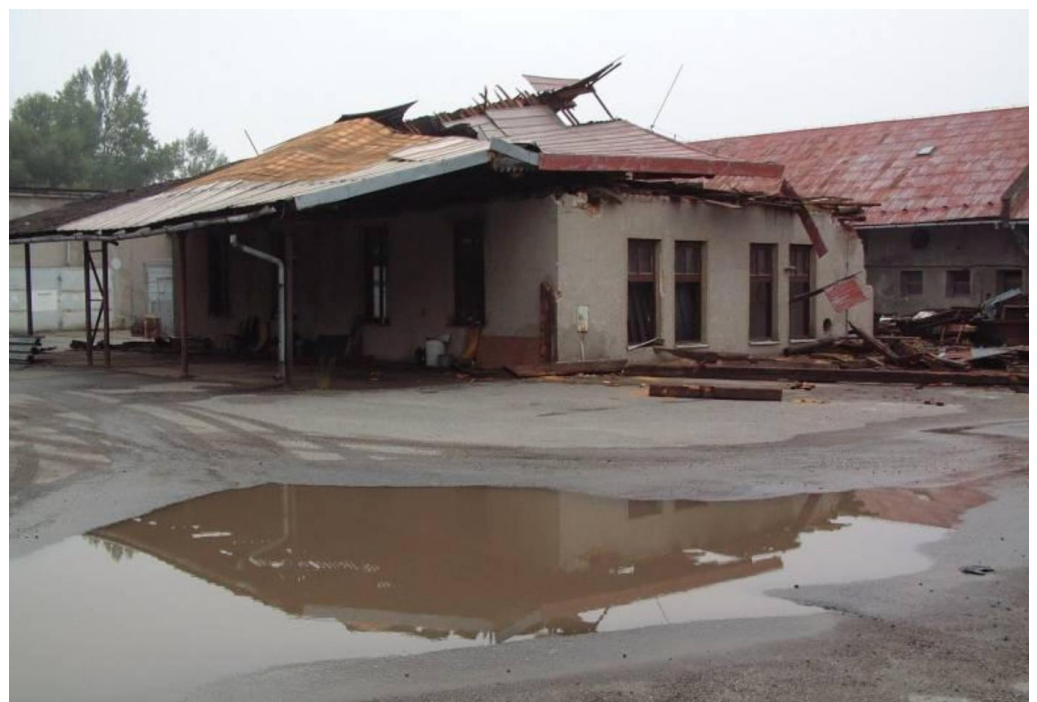
Figure 4. An example of a partially destroyed building from the grounds of a state farm. Source: [62].
