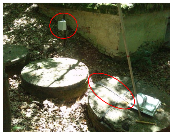
Fig. 11. Installed monitoring unit
