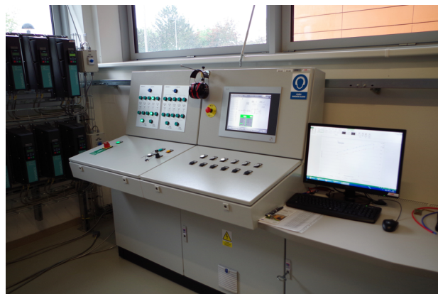
Figure 1. Controlling board for duct tract
