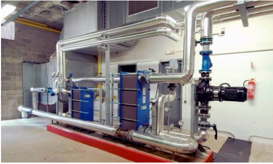
Fig. 6. Heat exchanger station
